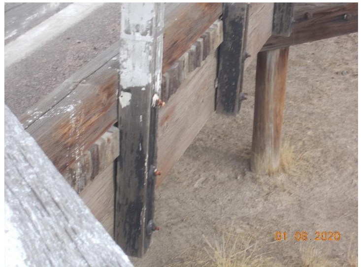
Paint sample M-21-J-LP02. The black paint is considered lead-based paint.
